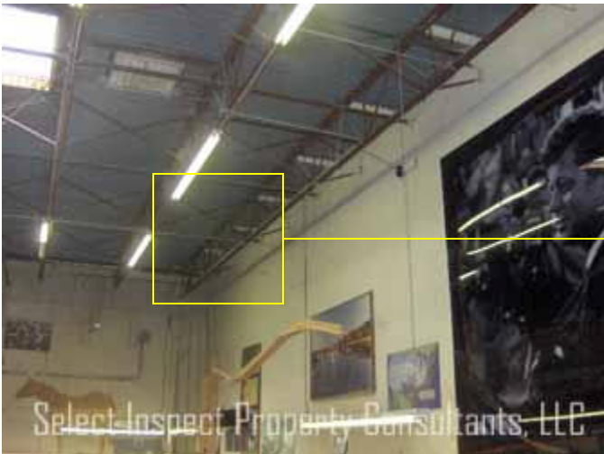
↑ workshop northeast; below condensate leakage discovered at roof; adjacent the raised roof section between office & warehouse/shop
