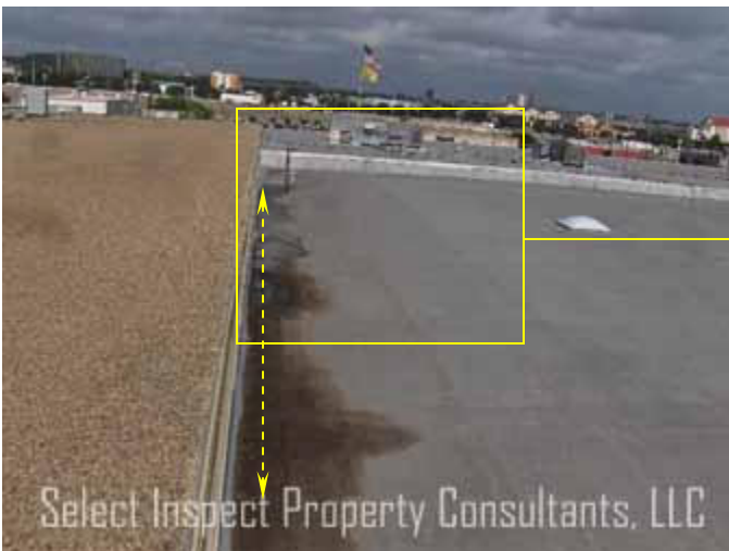
↑ south edge of the warehouse roof accumulating condensate & not draining adequately
