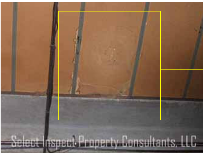
↑ warehouse west; below condensate leakage discovered at roof; adjacent the raised roof section between office & warehouse
