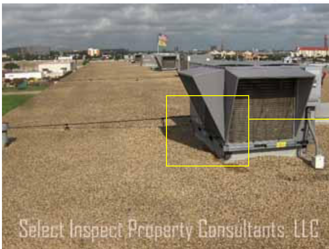
↑ air conditioning condensate leakage (& shadows) at southeast roof
