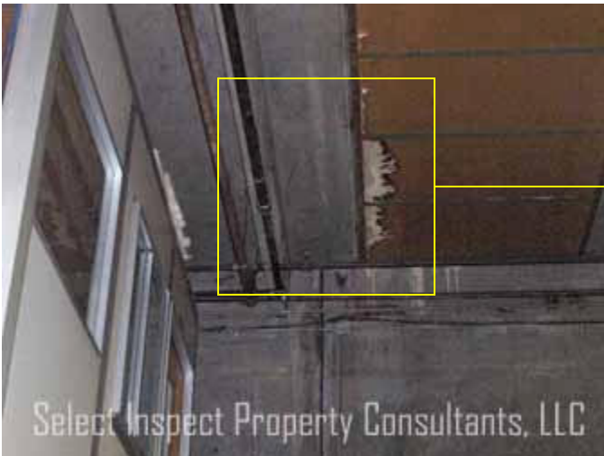
↑ warehouse northwest; stained ceiling, but Thermal imaging implies no anomalies; appears satisfactory
