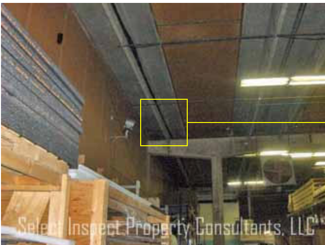
↑ warehouse west; below condensate leakage discovered at roof; adjacent the raised roof section between office & warehouse
