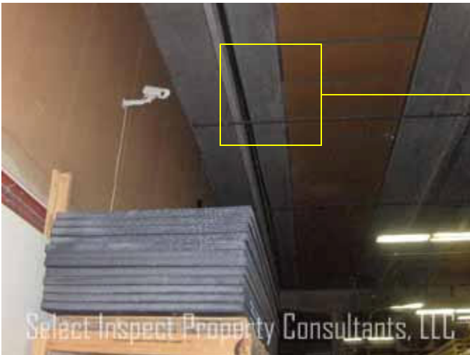
↑ warehouse west; below condensate leakage discovered at roof; adjacent the raised roof section between office & warehouse
