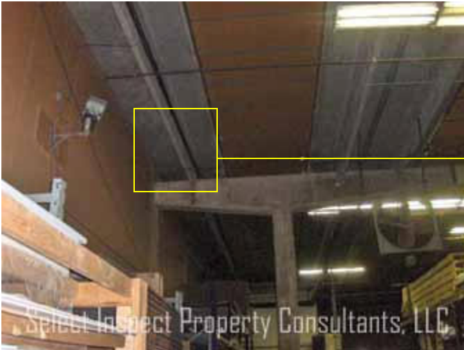
↑ warehouse west; below condensate leakage discovered at roof; adjacent the raised roof section between office & warehouse; same area as image above
