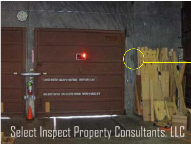
↑ chipped concrete wall & exposed reinforcement steel
