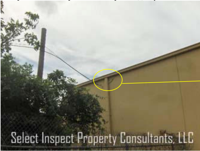
↑ cracked wall at the northeast
