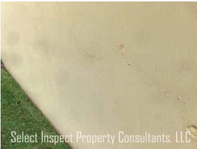
↑ stress cracks at southwest; sealed; Monitor; provide routine service, and maintain
