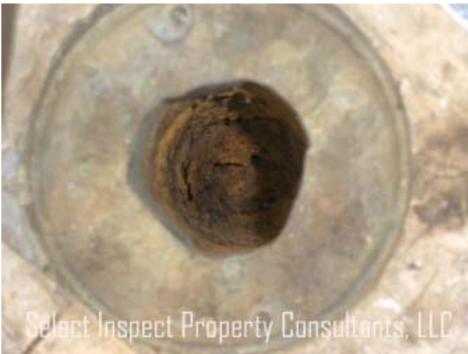
↑ excess corrosion within the upstairs bar floor drain.
