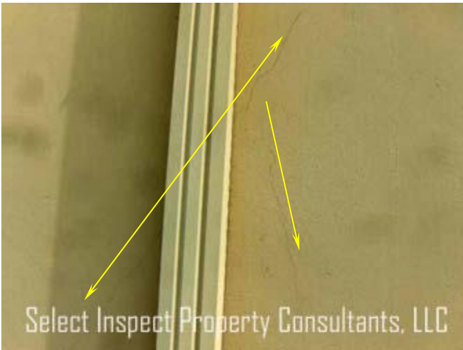
↑ stress cracks at southwest
