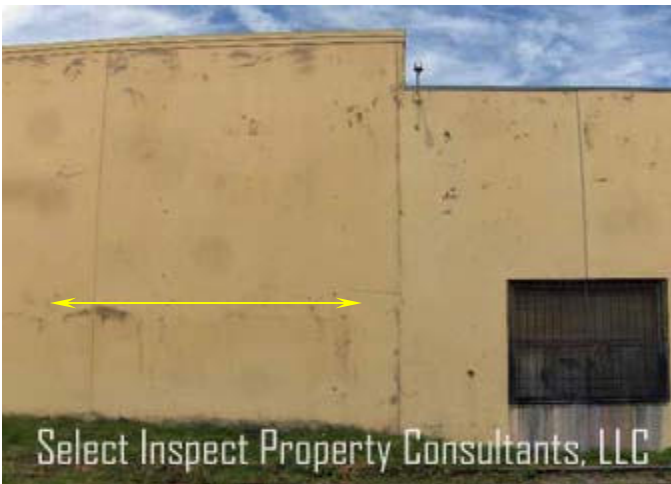
↑ stress cracks at the east
