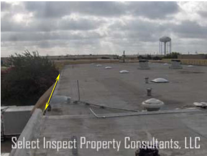
↑ inadequate slope & drainage of gutters at north
