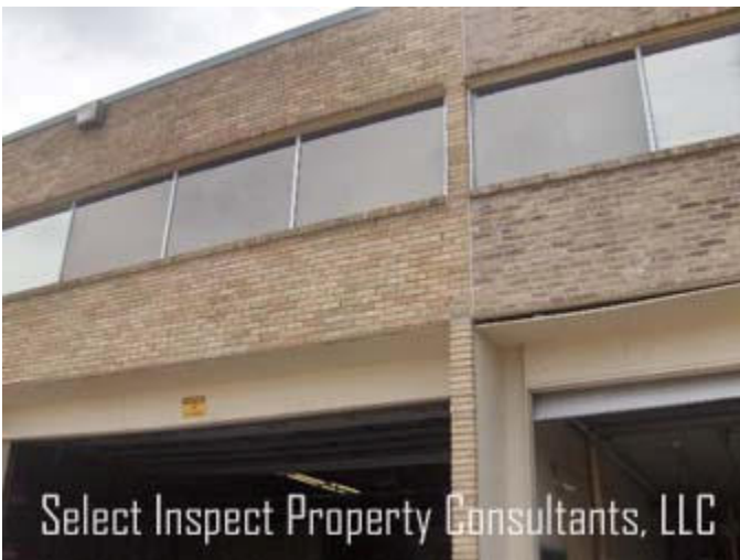
↑ cracked windows discovered at the gallery
