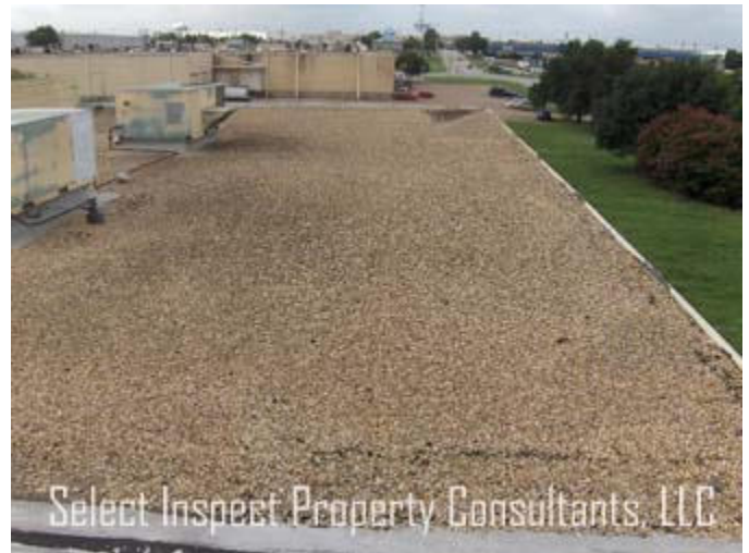
↑ shop roof front; workmanlike/in good order; Monitor; provide routine service, and maintain.
