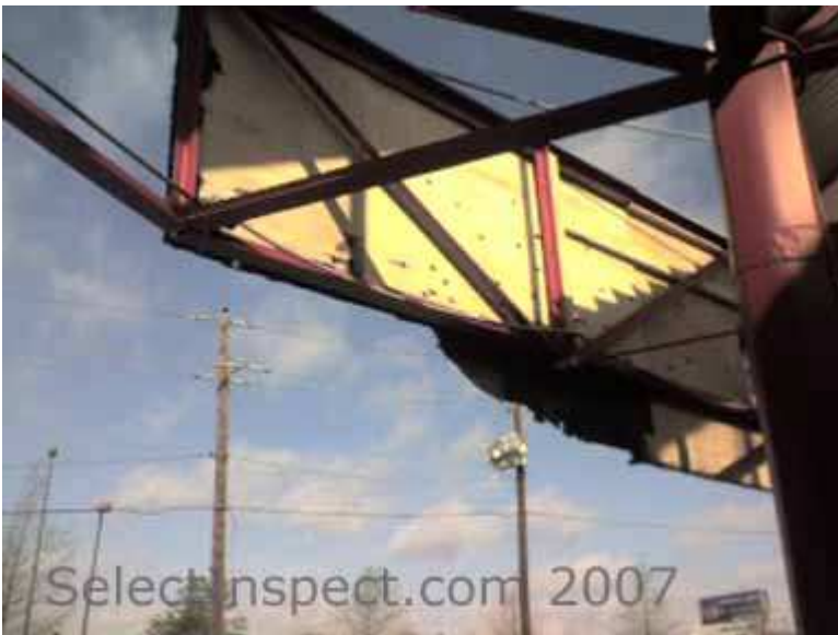
↑ deficient wood and stucco at sign structure- rear view
