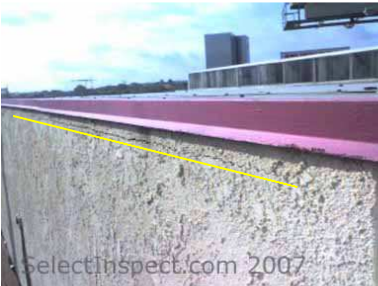
↑ horizontal cracking at east / rear area of bldg below roof parapet
