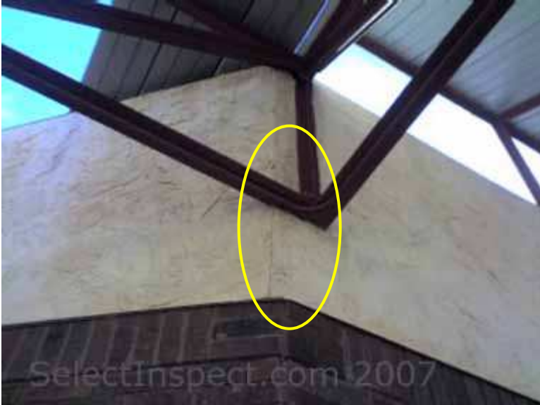
↑ moisture intrusion evidence and cracking at stucco- example
