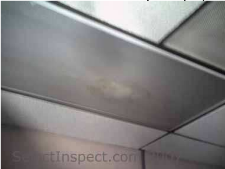
↑ moisture intrusion at light fixture in bathroom
