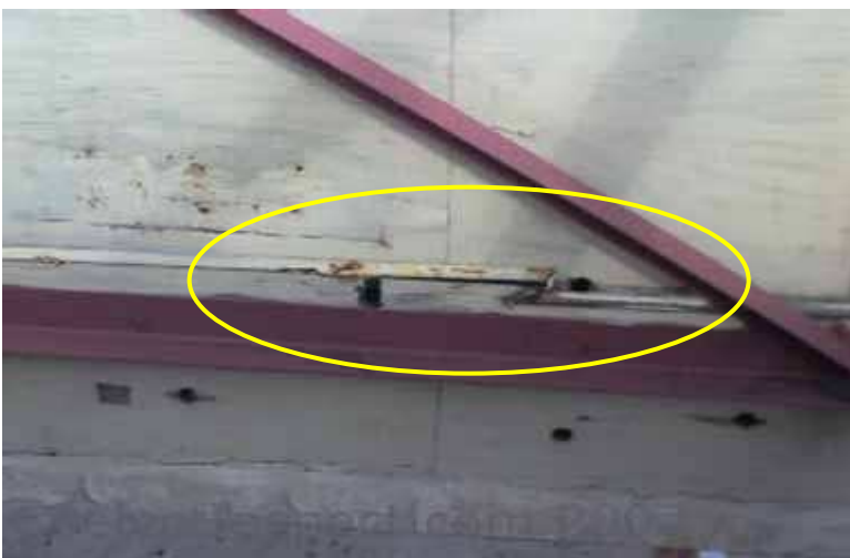
↑ amiss / deficient electrical at north behind sign structure
