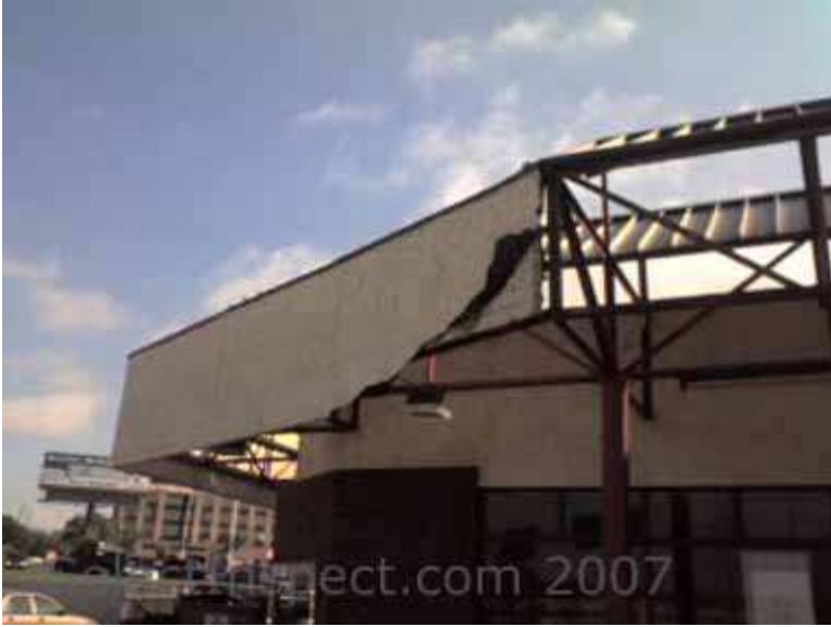
↑ deficient wood and stucco at sign structure- front view
