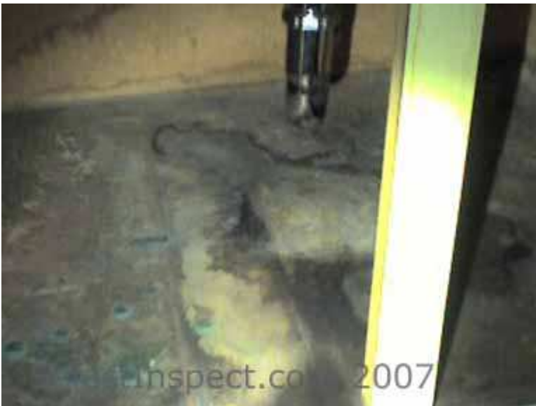
↑ moisture intrusion / fungus under breakroom sink
